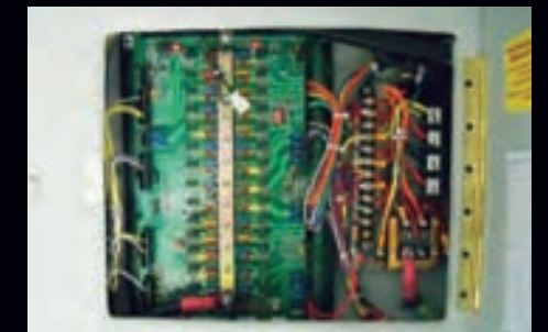
Printed electrical circuit board with LED trouble-shooting lights
